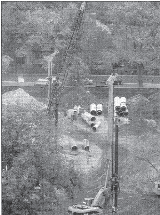
Construction is under way for the new Mather LifeWays continuing care retirement community towers at Davis Street and Hinman Avenue in Evanston. When finished, Mather North (11 stories) and South (10 stories) will include 243 independent living units in all.
